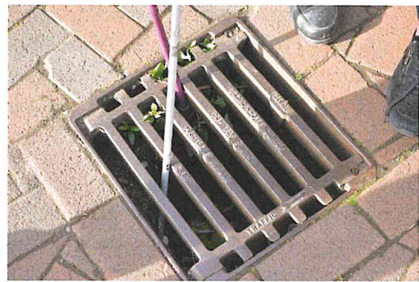
Figure 2 Drain cover in shared surface on Warbuton Way Long cane getting stuck
