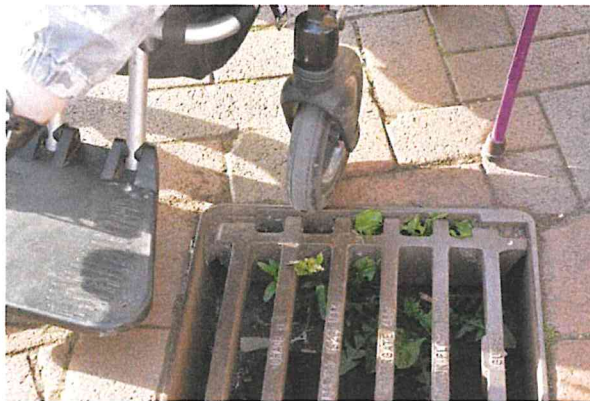
Figure 1 Drain cover in shared space on Warbuton Way
