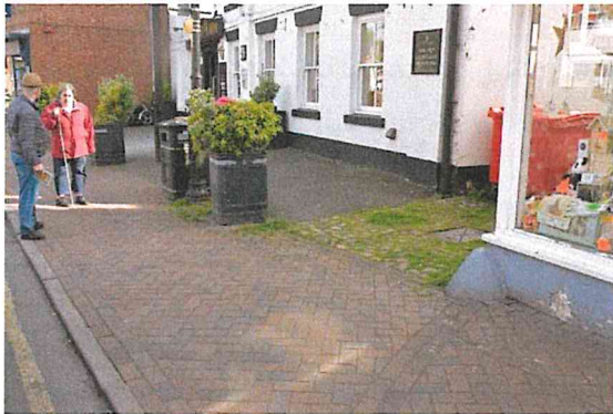
Figure 3 Tactile paving needed to indicate a hidden walkway
