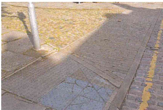
Figure 7 damaged tactile paving near DV8 Restaurant.
